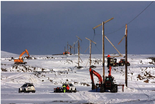
Fig. 7 Catastrophic failure in the north of Iceland, Kópaskerslína 1 (KS1) 10.09.2012.
